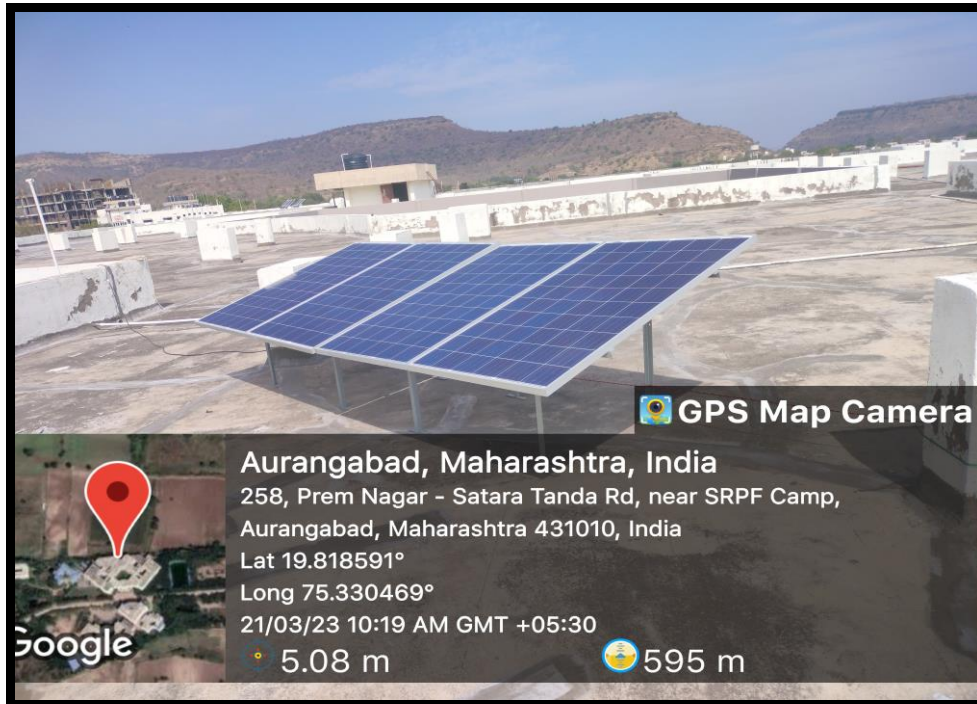
Fig. 1.2 Solar power plant of capacity 1.1 KWP installed on the rooftops of engineering building
