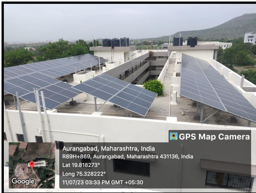
Fig. 7.1.2.1 Solar power plant of capacity 50 KWP installed on the rooftop boys' hostel building.
