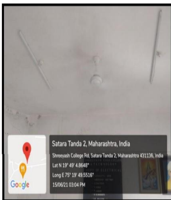
Fig. 3.1 LED tubes in the college premises
