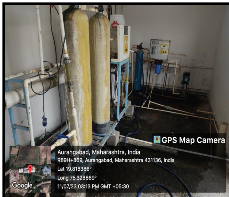
Fig. 7.1.4.5: RO Plant setup in the campus
