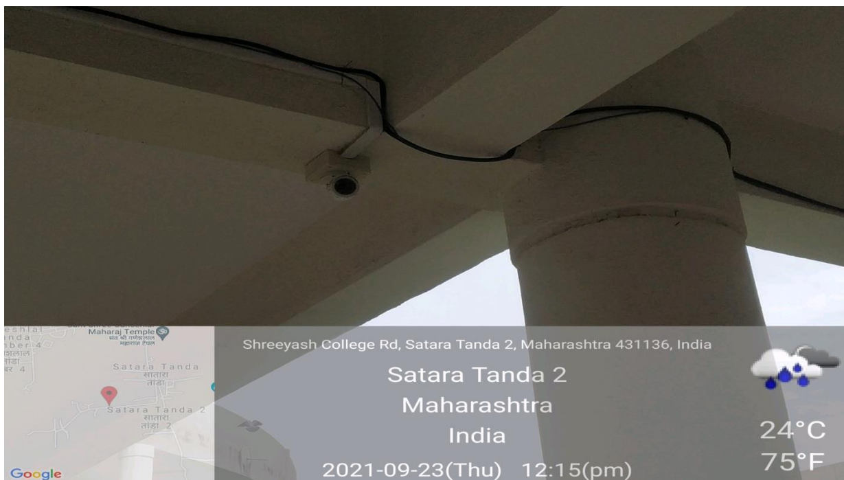
CCTV Camera (One of the Location)
